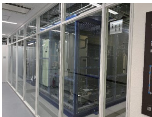
Hydrogen generation systems for Shimizu Corporation and Susumu Co., Ltd.
