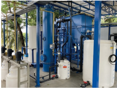
[Exterior of the system]
