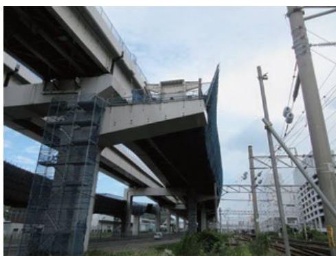
Elevated bridge of the Kurosaki West Bypass exit for the Kyushu Regional Development Bureau
