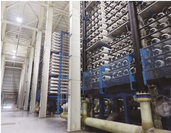
RO plant interior, seawater desalination plant in Qatar
