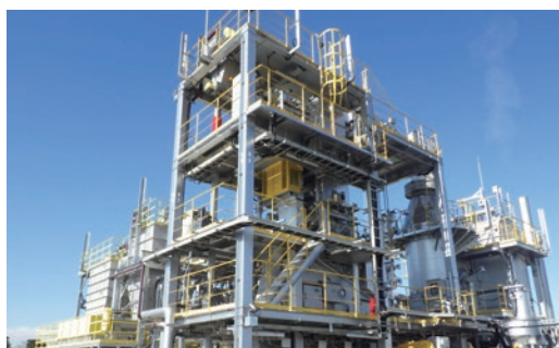
Demonstration test facilities
