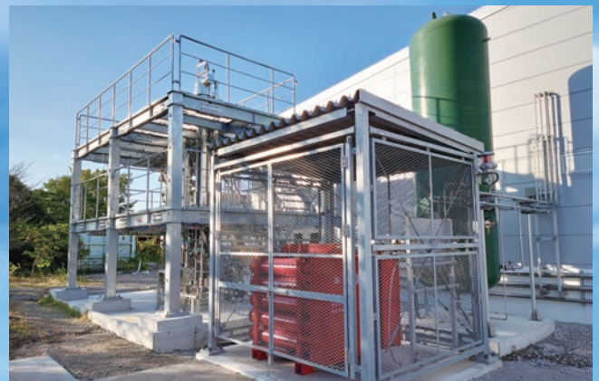
The PtG SQUARE demonstration facility
