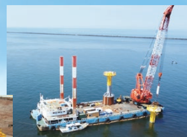
▲NEDO subsidized project: Offshore wind power generation low-cost construction technology development (suction-bucket construction technology demonstration); trial construction of demonstration foundation (Photo courtesy of Toyo Construction Co., Ltd.)
