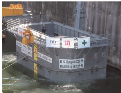
Tsuruda Dam (floating temporary closing facility)
