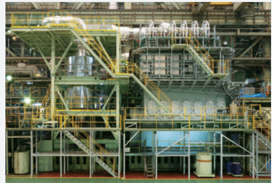
Marine diesel engine equipped with SCR system
