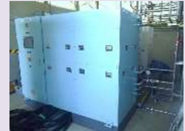
Hydrogen production system
