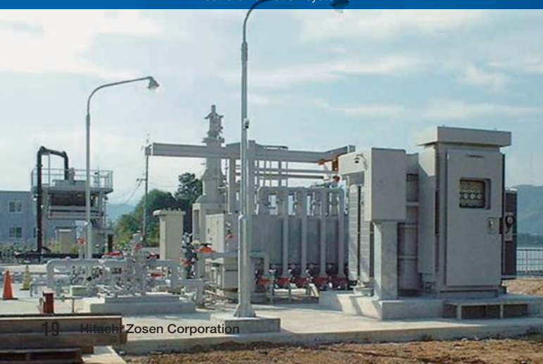
Electro chlorination systems
