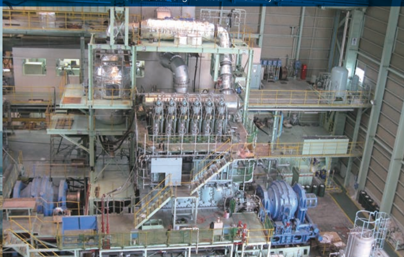
Marine diesel engine fitted with SCR system
