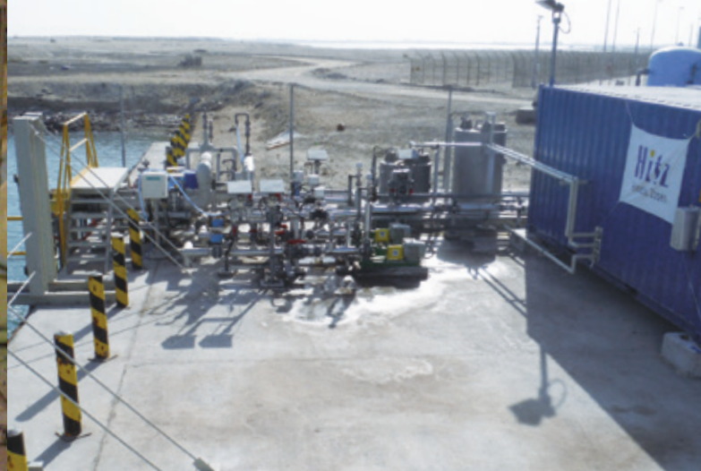
◀ Ibaraki Works No. 2 power generation
