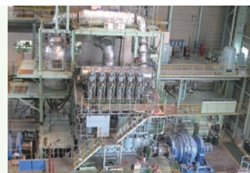
Marine diesel engine fitted with SCR system
