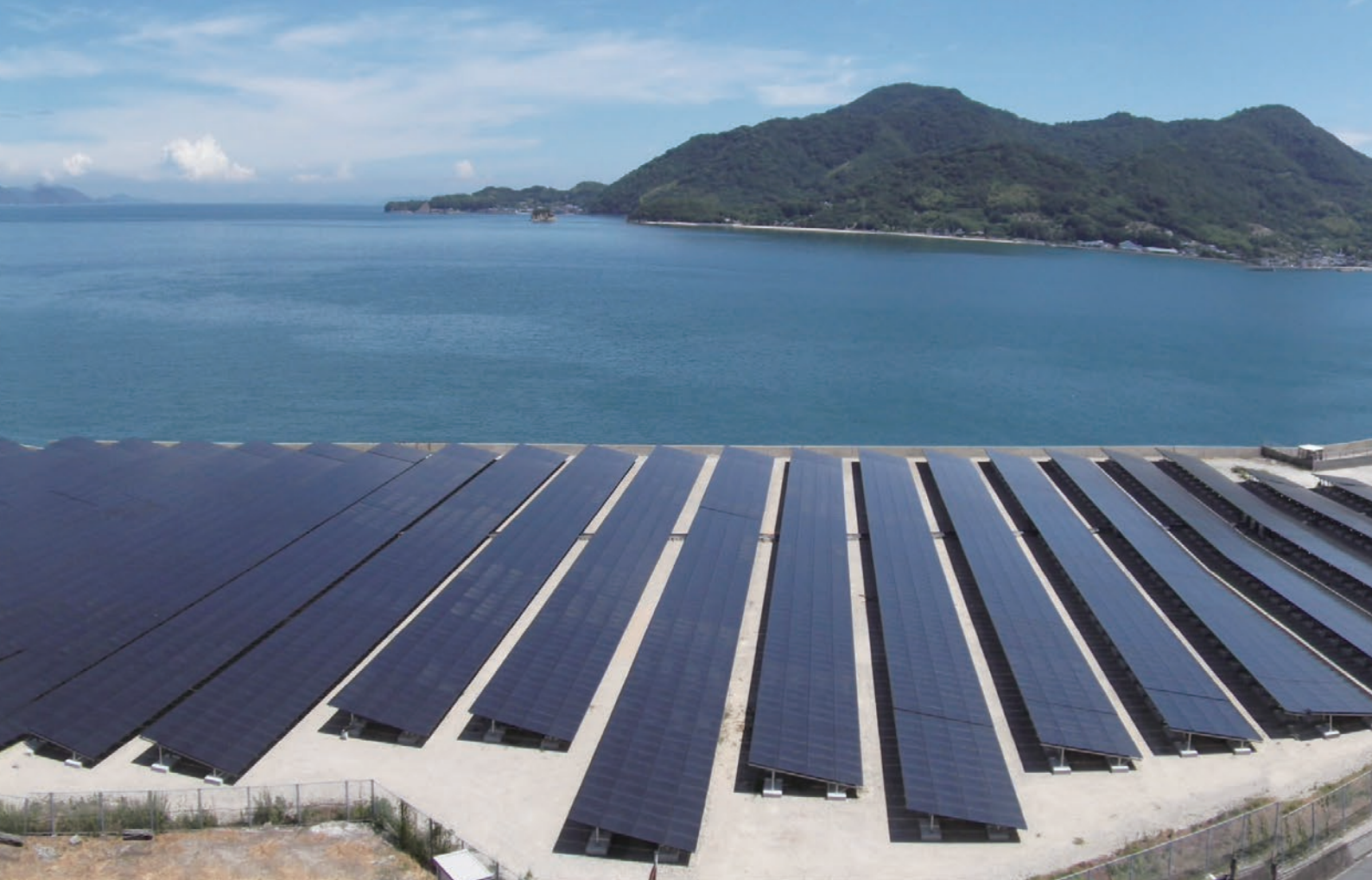
▲ Large-scale photovoltaic (mega solar) power plant in Innoshima Works
