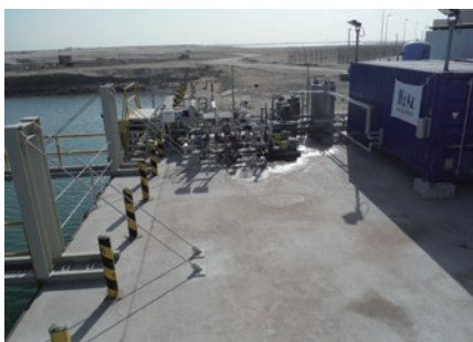
High-speed Seabed Infiltration System (Abu Dhabi demonstration plant)
