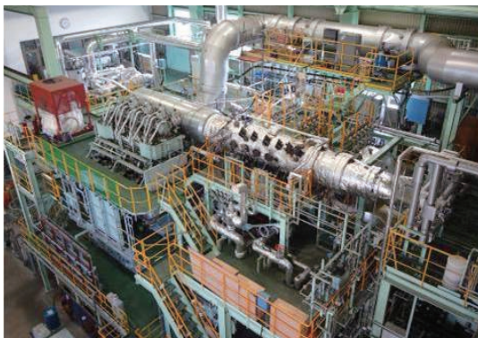
▲ Marine diesel engine fitted with SCR system
