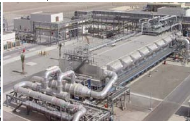
▼ Seawater desalination plant
