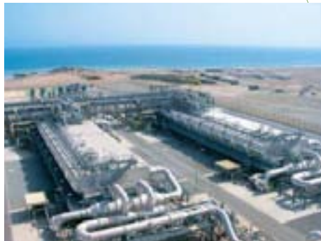
Seawater desalination plant
