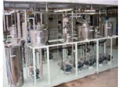
Continuous production system for biodiesel fuel
