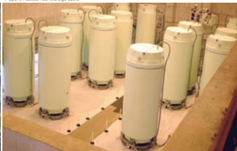
▼ Spent nuclear fuel storage casks
