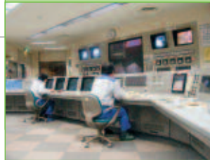
Central control office
