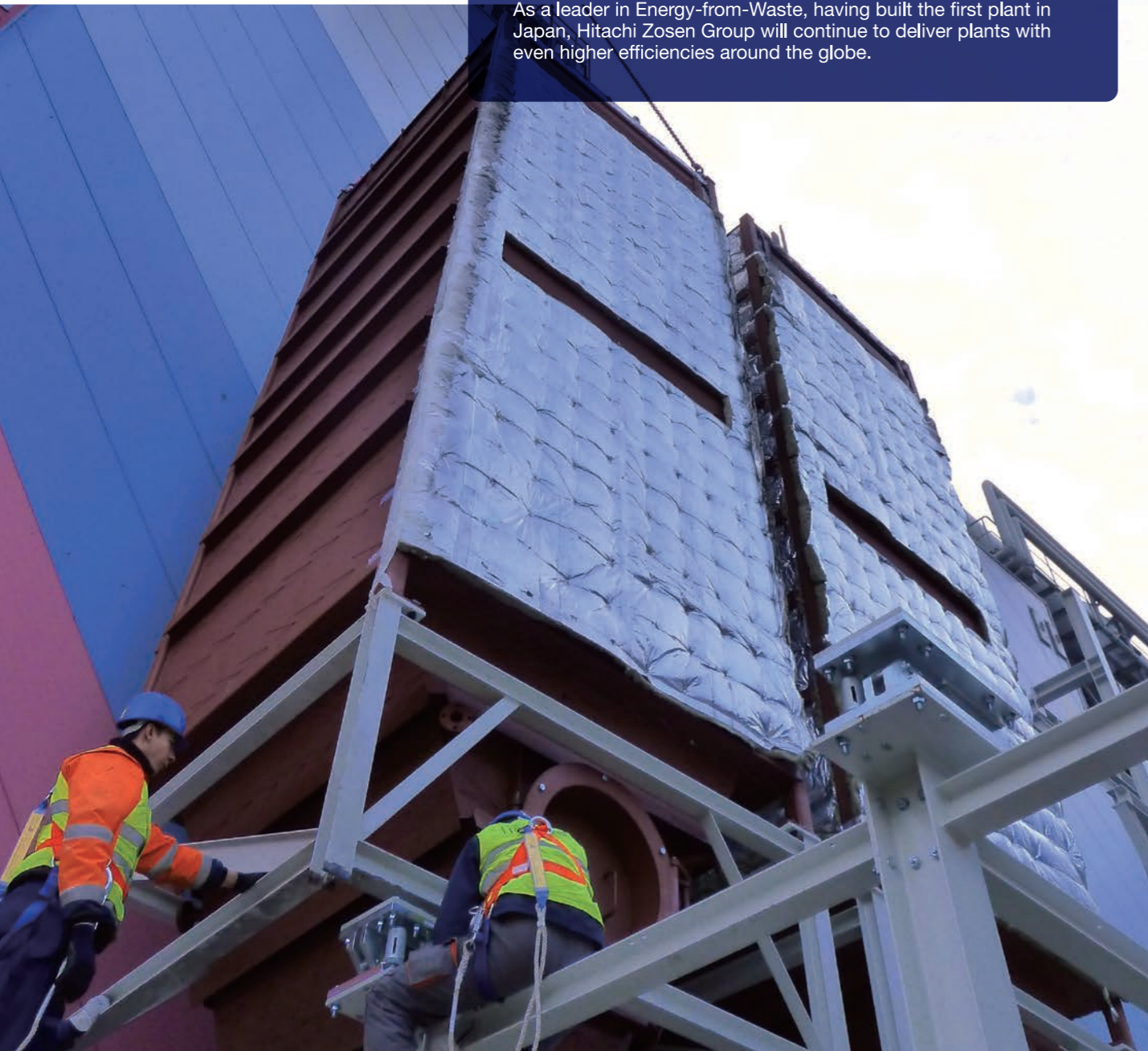
Energy from Waste Plant, Hinwil, Switzerland
