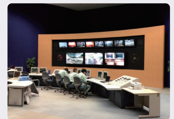
Rinkai Plant Central Control Room
